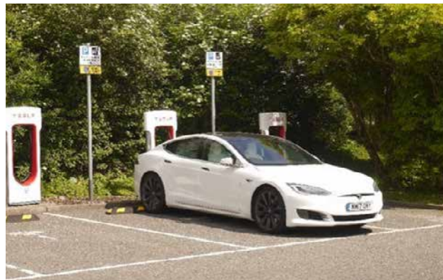
Figure 100: Example of electric vehicle charging points in a parking court.
