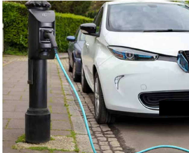
Figure 99: Example of on-street electric vehicle charging points.
